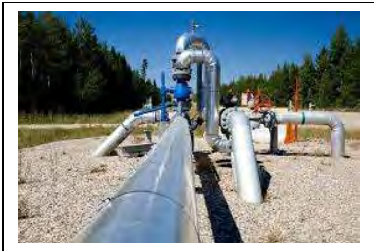
FIGURE 4-3. SIMULATED METHANE SOURCE: GAS-GATHERING PIPELINE ASSEMBLY
