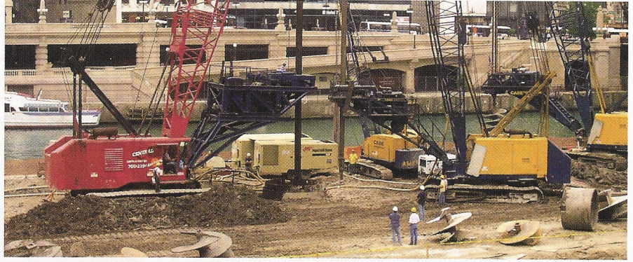
At the Trump International Tower jobsite in Chicago, IL, an oilier (left of crane operator) also assists in relaying signal messages to the operator. Procedures such as this can help keep the possibility of an accident to a minimum. While a crane operator can only accept signals from the signalman, anyone on site can give the operator an emergency stop command. (Photo by Peter J. Gallanis)
