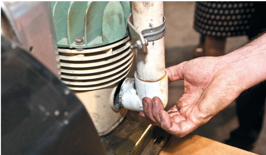
The connection between the snorkel and the compressor was not secure, which would allow carbon monoxide to freely enter the compressor.
